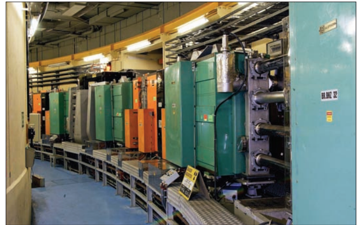
Fig. 1. One of the 16 magnet periods in the PSB tunnel. Right to left (following the beam): a bending magnet (dipole, green); an empty straight section with four superposed vacuum chambers; a bending magnet; a quadrupole triplet (focusing-defocusing-focusing, orange); a bending magnet; and RF equipment for beam acceleration (grey) in the next straight section.
